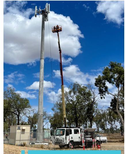
The new Digital Connectivity tower was wired in October and is now live, doubling capacity in Moranbah.
